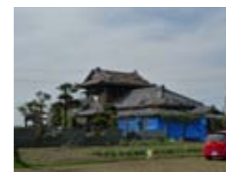
Photo 16 Damage to tile roofing
