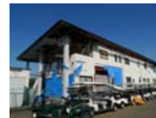
Photo 7 Damage to golf-course clubhouse
