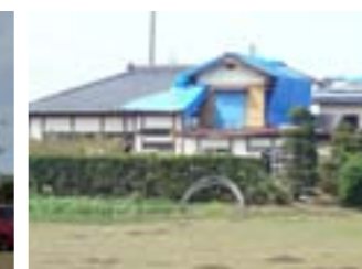
Photo 17 Damage to tile roofing and exterior walls
