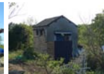
Photo 9 Damage to conventional wood-frame structure
