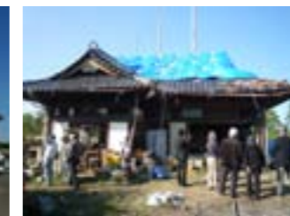
Photo 8 Damage to traditional wood-frame building
