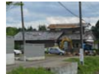
Photo 4 Damage to conventional wood-frame building (1)
