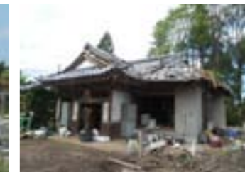
Photo 6 Damage to traditional wood-frame building
