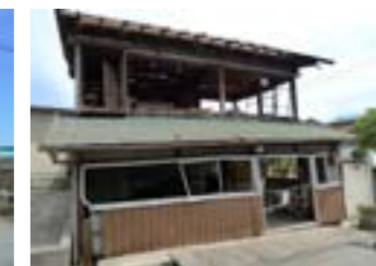
Photo 15 A standing structure tilted and horizontally shifted from its foundation
