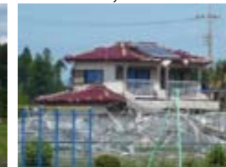
Photo 5 Damage to conventional wood-frame building (2)
