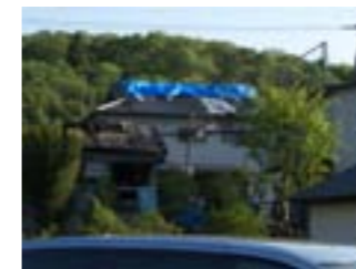
Photo 10 Damage to tile roof
