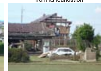
Photo 18 Damage to wooden roof truss section
