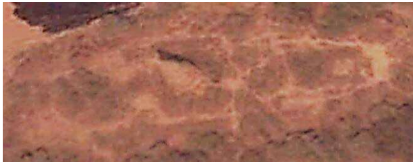
Before repair (Google earth 2010.3.20 shooting)
